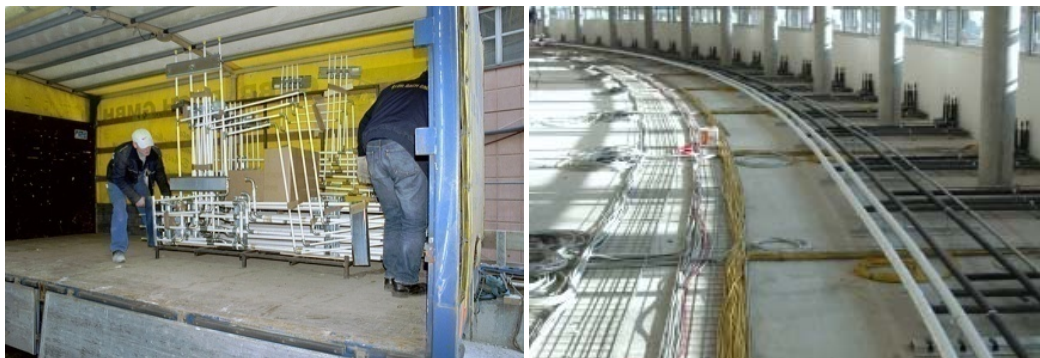
Figure 2: pre-packaged materials for MEP-system installation (left hand side); installed MEP systems (right hand side).
